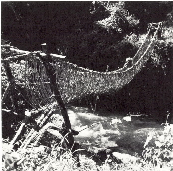
Fig. 15. A primitive hanging bridge in the north-eastern Bhutan Himalaya. This bridge is built in a primitive way, only by liana and bamboo, a system over 2000 years old. (Fot. A. Gansser).
